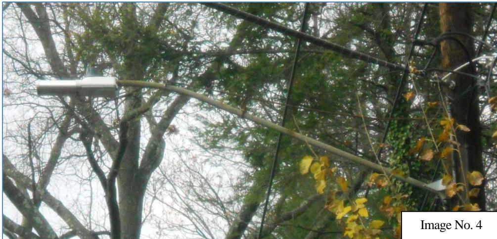
LED streetlight installed on Dorset Avenue in the Town of Somerset
